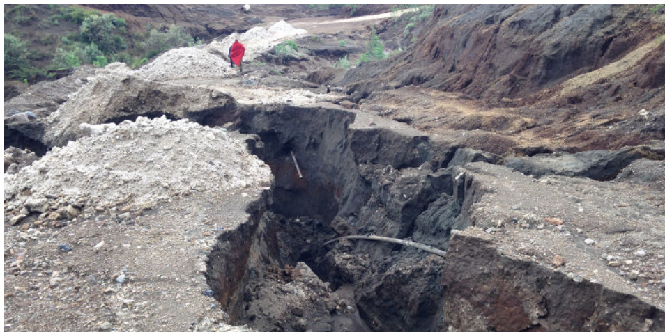
Broken water pipes at resettlement area
